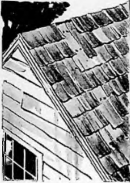
A damaged roof shows first signs of decay
